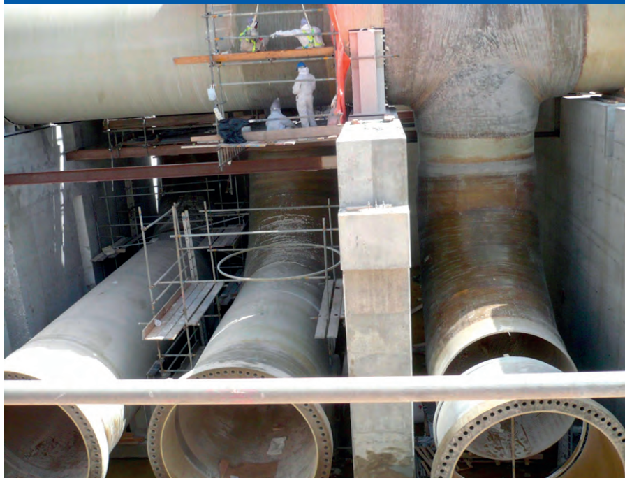
Future Pipe Industries
