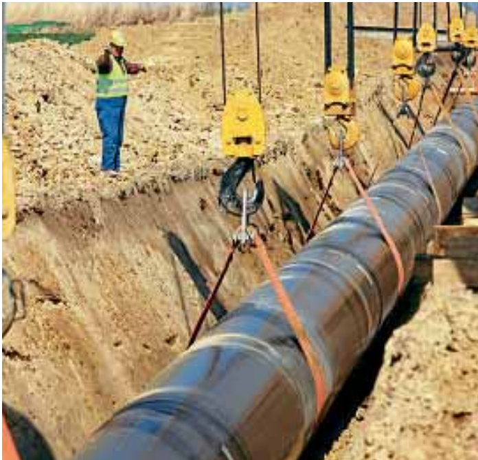
Traditional high-grade steel is being replaced by fibreglass piping.
