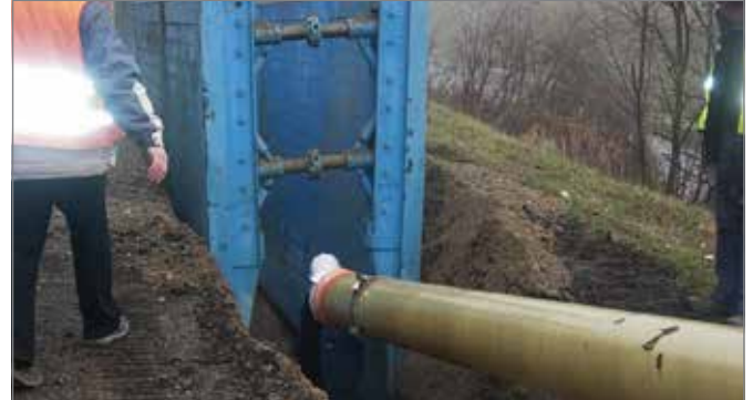
Fig. 6.1. Trench in unstable soil
