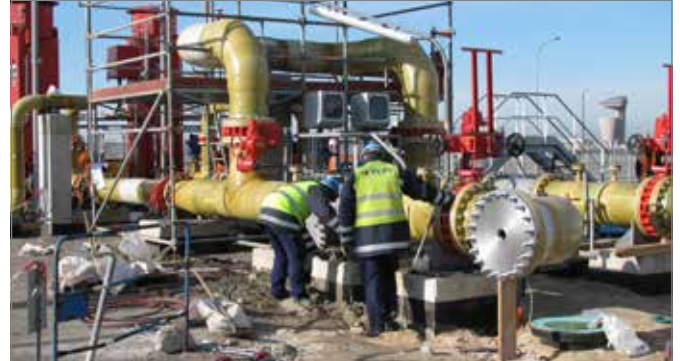
Fig. 7.1. Aboveground pipe system
