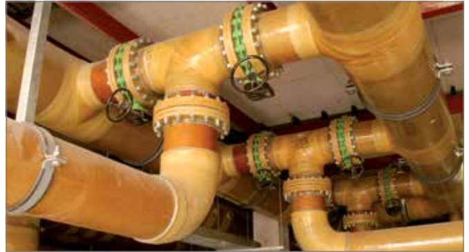
Fig. 7.7. Overhead supported pipeline
